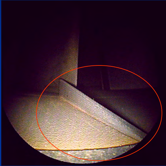
Stage S-1 Shim Protruding Into Air Path
