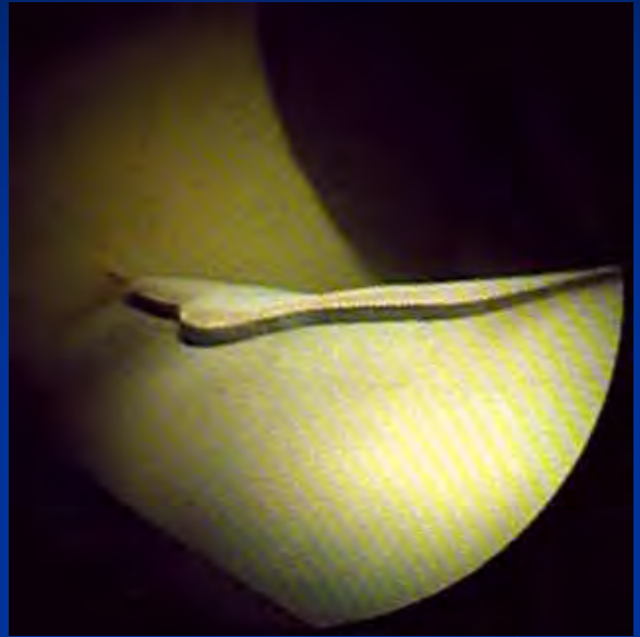
Cracked Transition Piece
