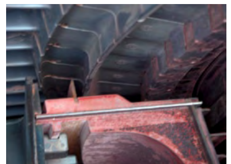
2-3. Dimensional checks pinpoint deformation and other problems that should be addressed in your repair spec (below)
